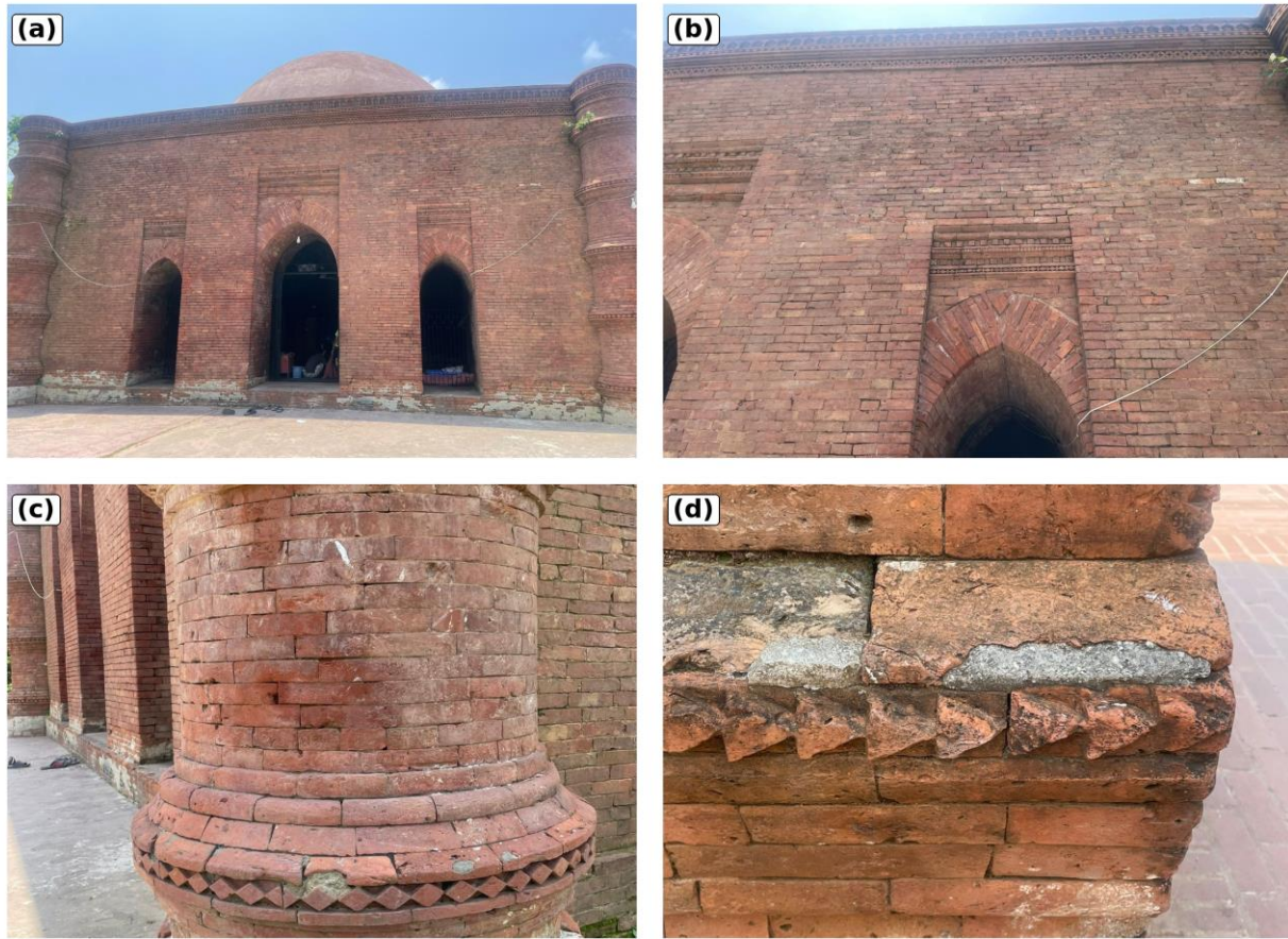
Figure 5. Singair Mosque: (a) overall facade; (b) entrance/cornice field; (c) corner-turret serial mouldings; and (d) close view showing chipped or missing units and local infill. Photographs by the author, 2 April 2026.
