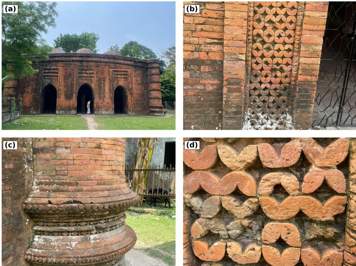
Figure 4. Nine-Dome Mosque: (a) overall facade; (b) doorway-adjacent repetitive decorative panel; (c) corner-turret molded bands; and (d) close view showing broken, eroded, or missing units and local discontinuity. Photographs by the author, 2 April 2026.
